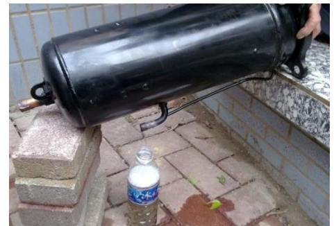
Figure 5-4.14: Draining oil from a compressor
